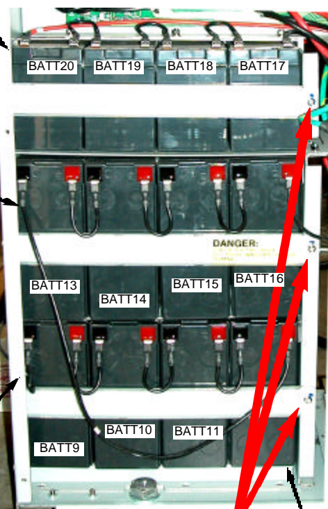
LEFT SIDE BATTERY DETAIL
