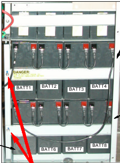
RIGHT SIDE BATTERY DETAIL
